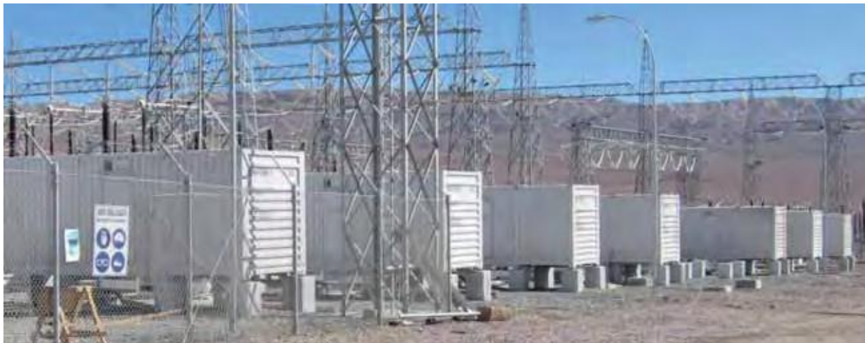
Figure 3-3 | Li-ion battery supplying up to 12 MW of power at Los Andes substation in Chile (A123, 2009)
