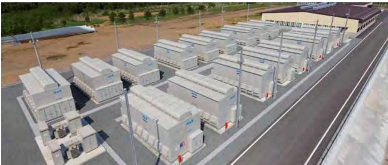
Figure 3-10 | NaS battery units – 34 MW (Japan Wind Development Co.)
