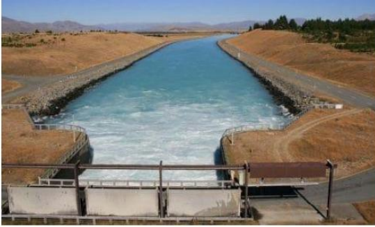
Fig 3: Power Canal of Lake Tekapo, Newzeland
